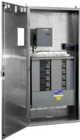
PowerLogic E4800 meter as part of an integrated power center (IPC).
