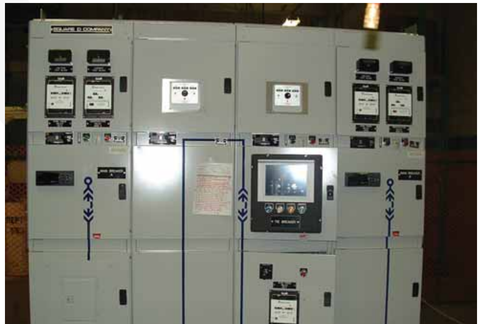
Square D equipment provided tracking and monitoring functionality but also load control the starts generators and drops low priority demand.
